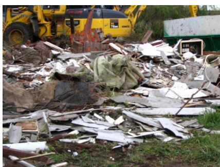
Inappropriate disposal and removal of asbestos cement material
